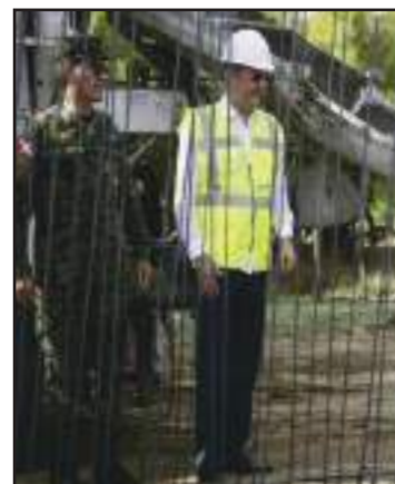
Dominican President Luis Abinader visiting a wall being built at the border between the two countries.
